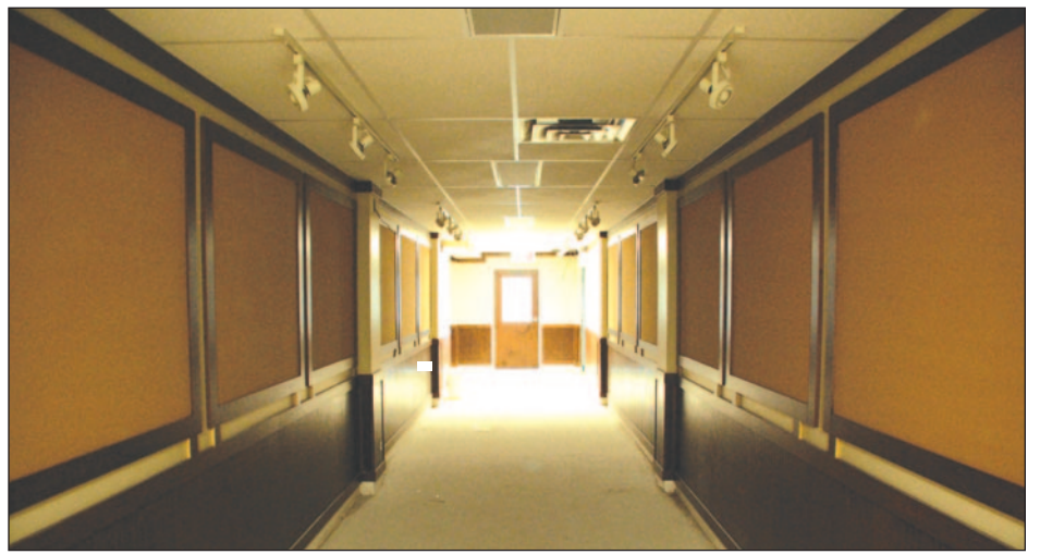
Downstairs, both locker rooms have been extensively revamped, beginning with the excavation of the basement to provide more headroom and airier atmosphere. The walls are now covered in wainscoting, giving the area a classic look. Bathrooms upstairs have been refinished in granite.
