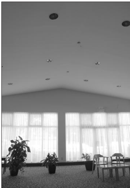
The ceilings in the dining room and lounge have undergone dramatic facelifts, with more insulation and new lighting as well as structural improvements.
